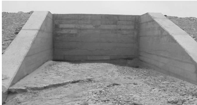
Figure 7.1 Fully blocked outlet of the Wadi Laba culvert
