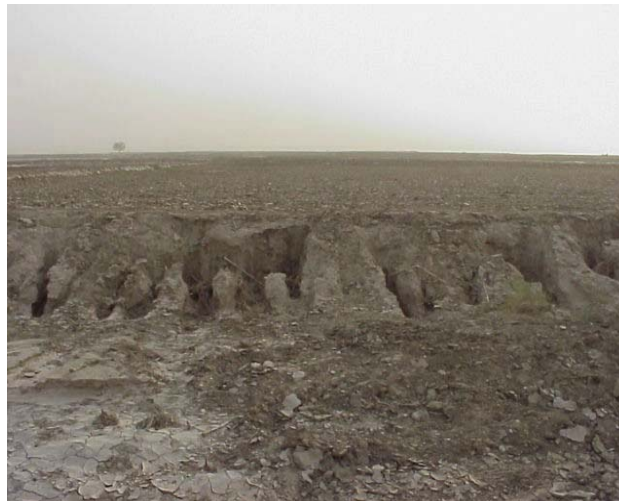
Figure 3.4 Severely eroded field bund in Wadi Laba, Eritrea
