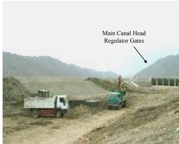
Figure 4.11 The Wadi Laba gravel trap with the cleaning operation in action
